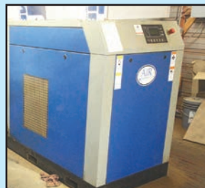
40 HP SHANGHI AIR COMPRESSOR
